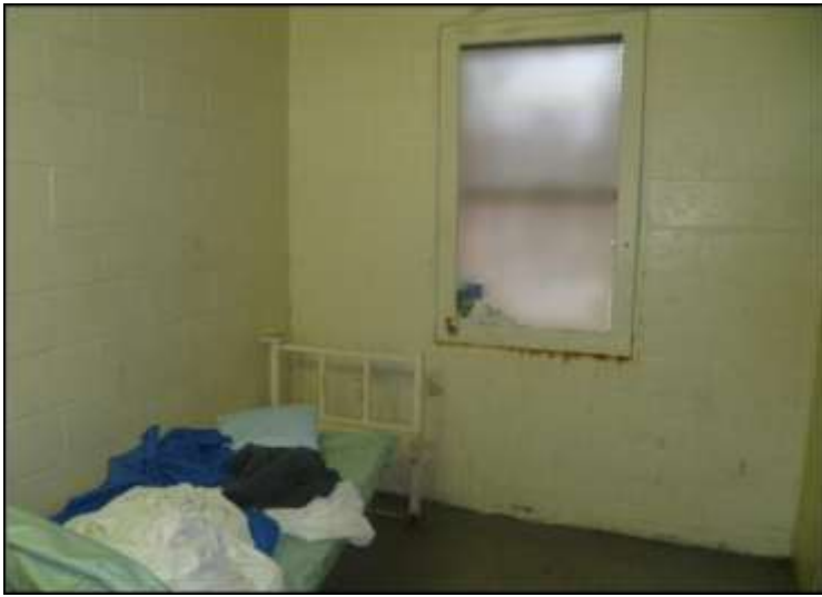
Occupied cell - metal bed to be replaced
