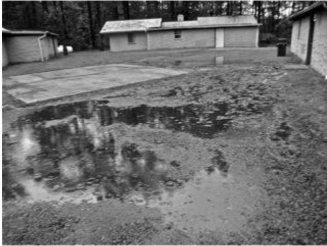
Standing water at Morning Star
