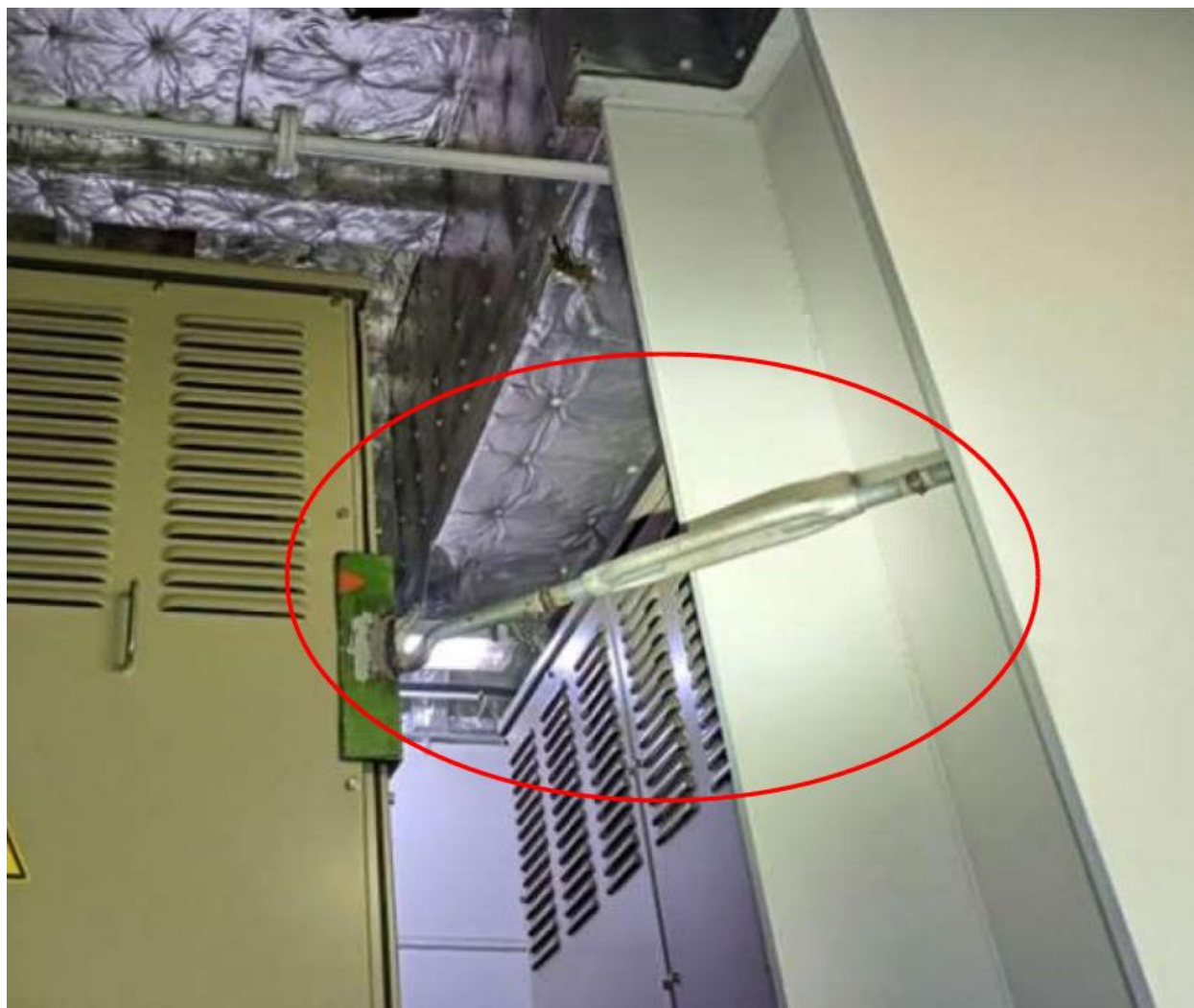
The photo above depicts an improvised “tumbuckle” being used to dampen vibration on one of the DALI’s transformers.
